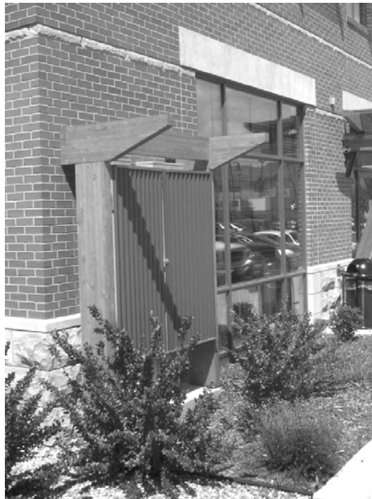
Figure 65 – It is appropriate to integrate equipment panels into the building design.
